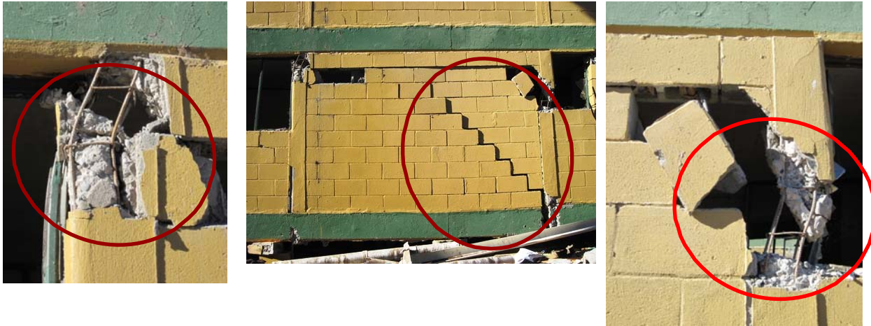
Figure 7. Failure of RC tie-columns caused by the shear failure of the masonry wall panel.
