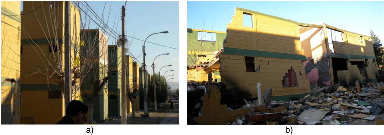
Figure 9. Collapse of a three-story confined masonry building in Santa Cruz: a) building complex, and b) a building that collapsed at the ground floor level.
