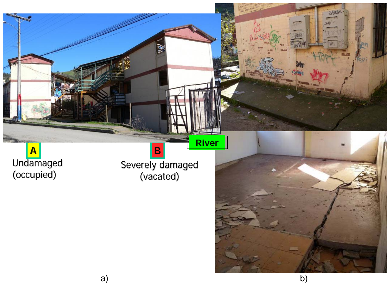
Figure 18. A building in Constitución experienced severe damage: a) building B located closest to the creek located on the right side of the building, and b) extensive exterior and interior damage in the building.
