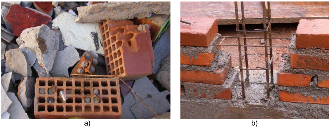
Figure 3. Confined masonry construction: a) a typical hollow clay unit, and b) a toothed wall-to-tie-column interface.
