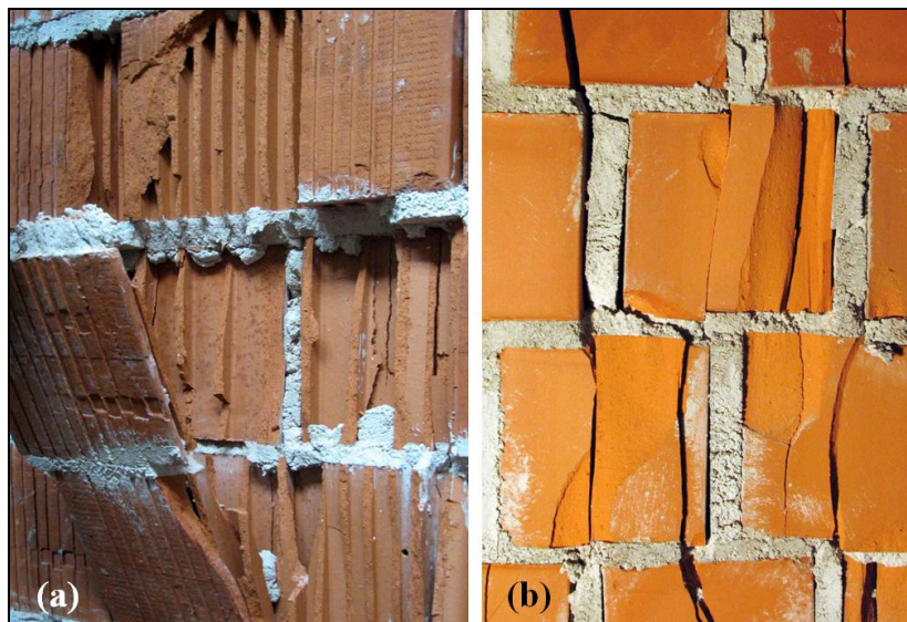
Figure 9. Details of failure mechanisms at compression. a) Buckling of shells in the case of the hollow block B4. b) vertical cracking of units B6
