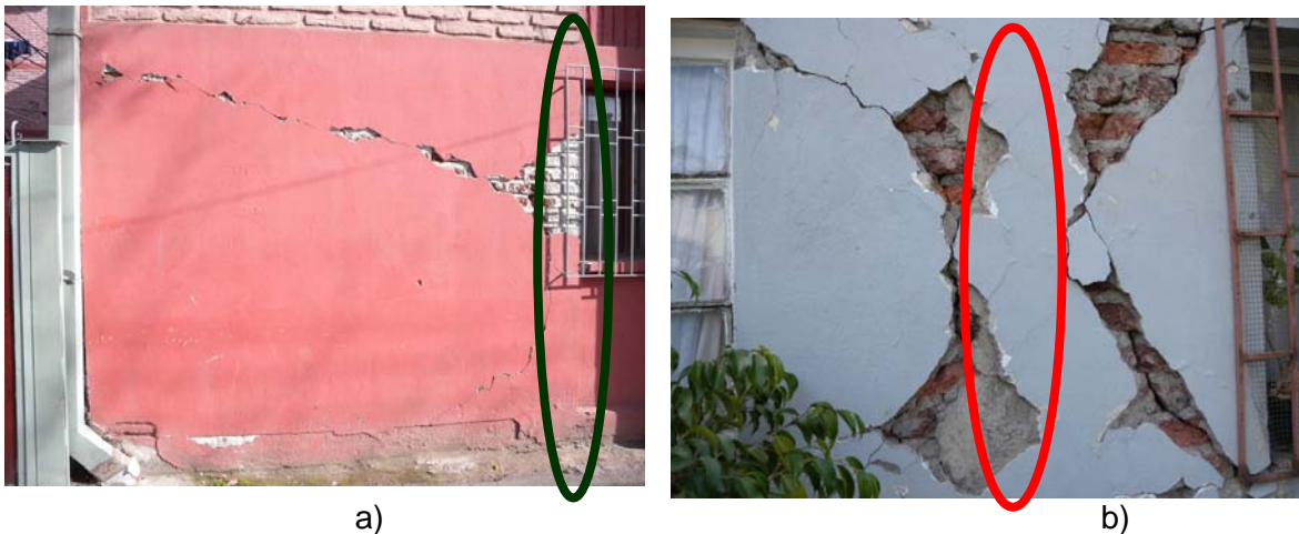
Figure 17. In-plane shear cracking of piers in brick masonry walls: a) a confined masonry panel with RC tie-columns at both ends (note RC tie-column highlighted with a black ellipse), and b) an unconfined panel (note RC tie-column at the middle of the pier highlighted with a red ellipse).
