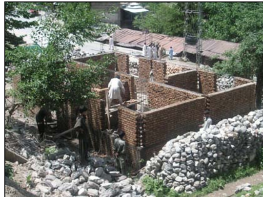
Fig. 4: Raising wall from sill to lintel band before pouring of the tie-columns
