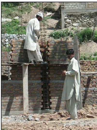
Fig. 5: To ensure proper filling of the tie-column it would have been better to fill the lower part of the tie-column together with the sill band
