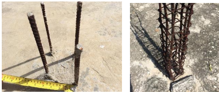
Fig. 7 – Left – Existing column extension with (3) #4 and (1) #3 bars Right – Existing column extension with smooth rebar and stirrups already placed
