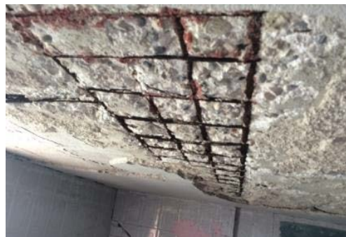
Fig. 8 - Existing slab in poor condition
