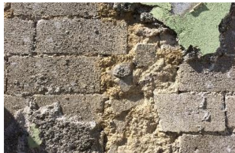
Fig. 6 – Poorly repaired wall crack
